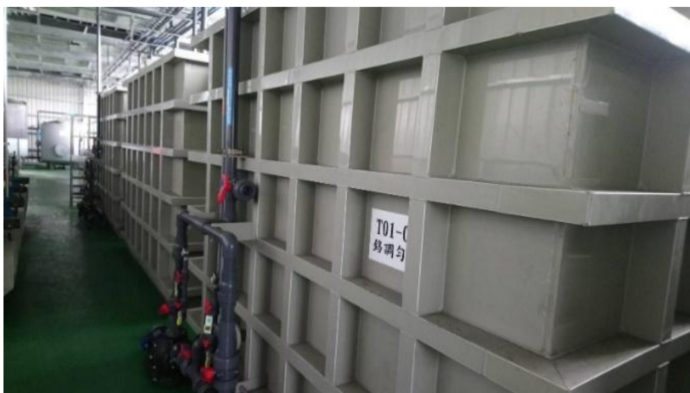
Wastewater Treatment System at the Second Factory
